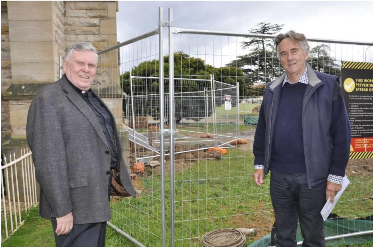
Dean Phillip Saunders and heritage architect Michael Fox show the excavations underway on the Cathedral's eastern aspect. Photo: Louise Thrower.
